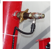
Hydraulic Sensor Installation
